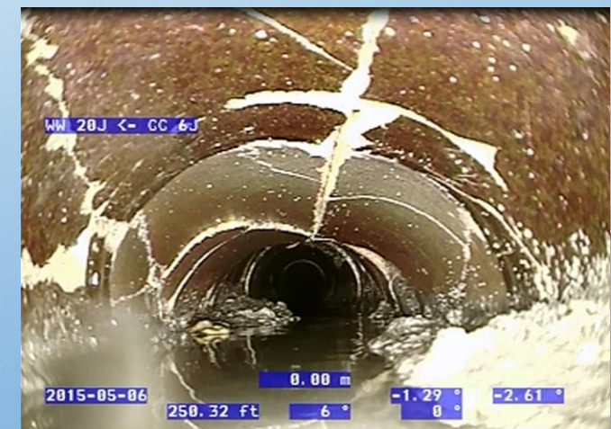
Broken and collapsing pipe
