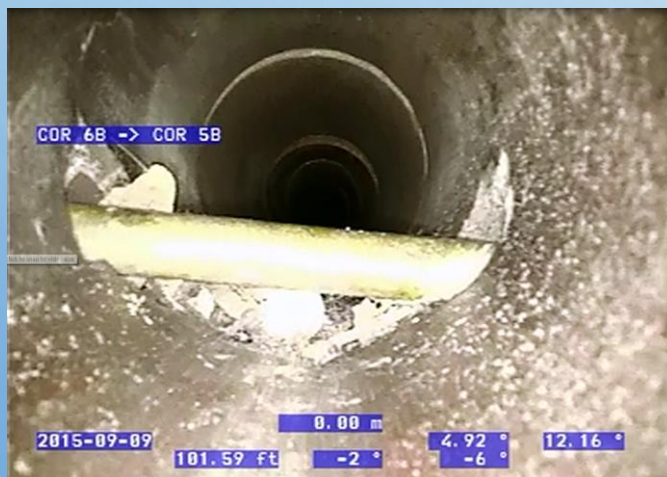
Natural Gas service line drilled through pipe
