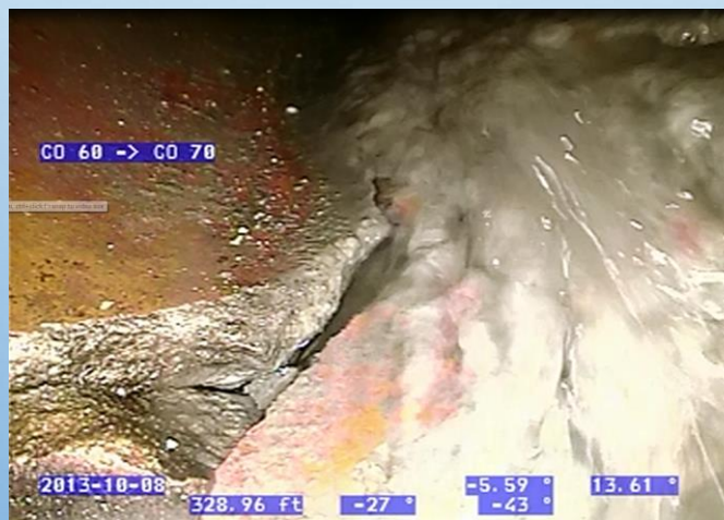
Broken pipe with infiltration
