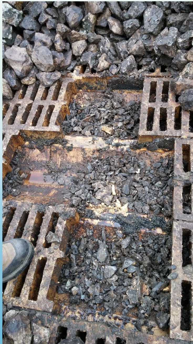
Lake St. – Trickling Filter media and underdrain
