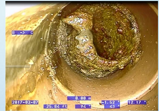
FOG (Fats, Oils, & Grease) in Lateral Connection
