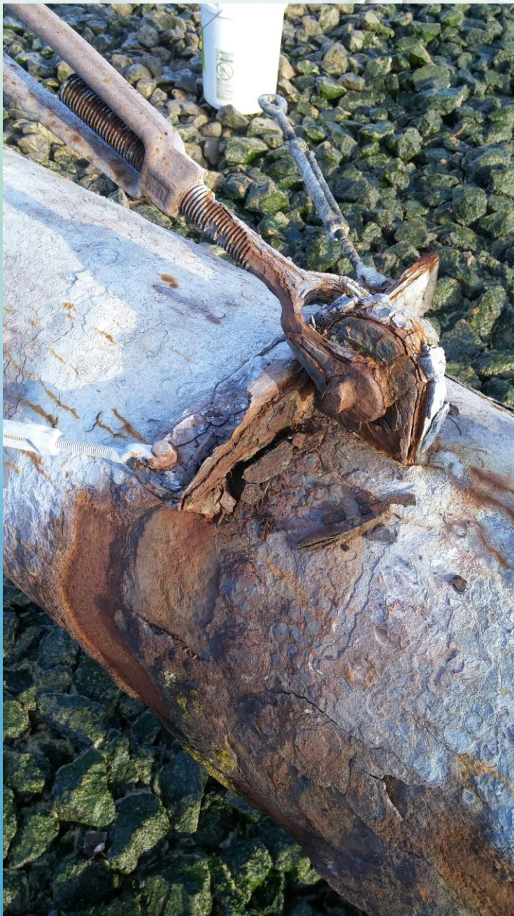
Lake St. – Trickling Filter distribution arms
