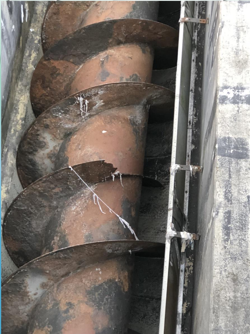
Milton St. – Influent Archimedes Screw Pump
